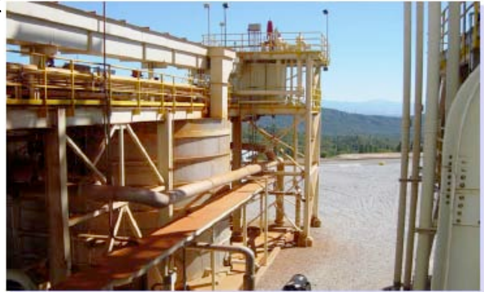
Photo 6: Part of the lime neutralization/high-density sludge acid mine drainage treatment plant at Minnesota Flats. The large tank at center-left is one of two in which acid mine drainage is mixed with lime slurry.
